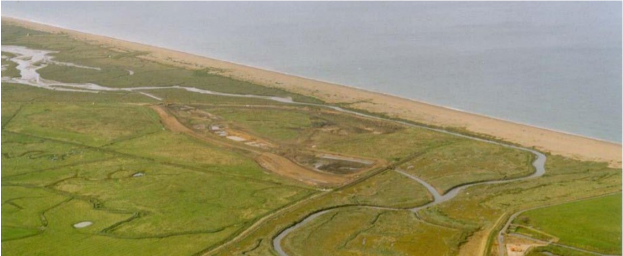
Construction of River Glaven managed realignment behind the Cley to Salthouse shingle barrier. Source: https://www.therrc.co.uk/sites/default/files/projects/47_northnorfolk.pdf
